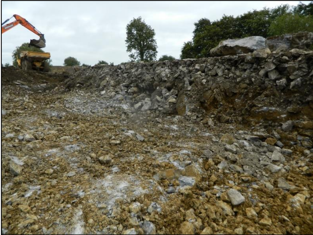
Plate 28 Facing east showing broken stone fill in north-facing section of excavation for stage 2 channel
