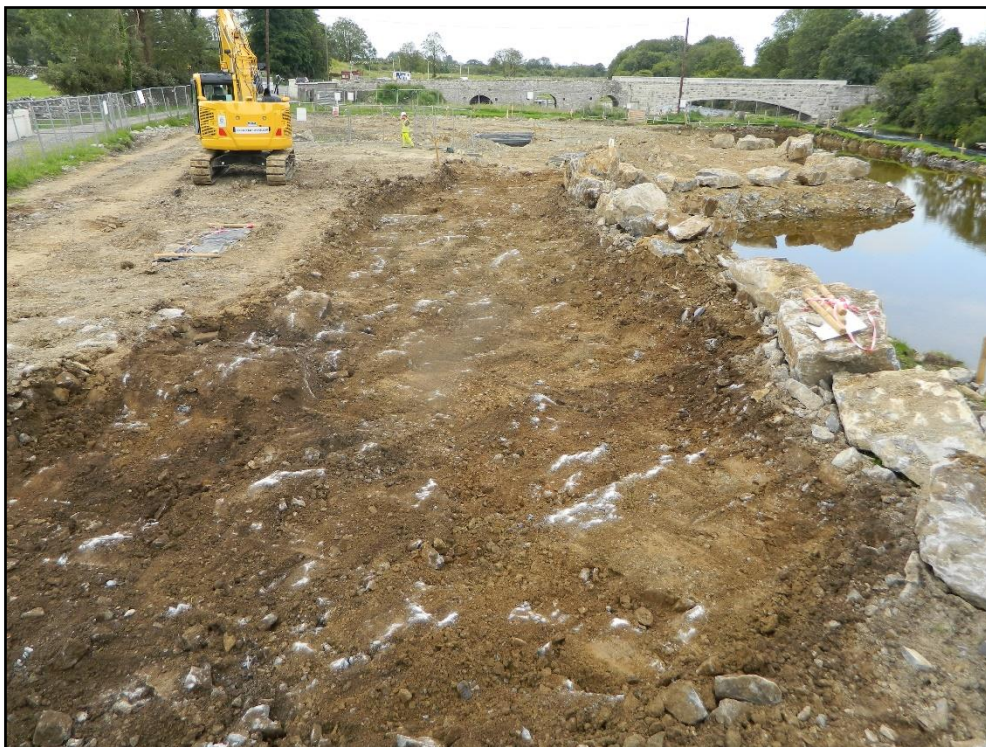
Plate 27 Facing WSW showing final site clearance with SK15 (under cover) left of centre
